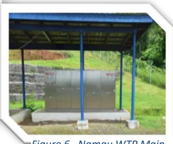
Figure 6. Namau WTP Main switchboard and shed.
