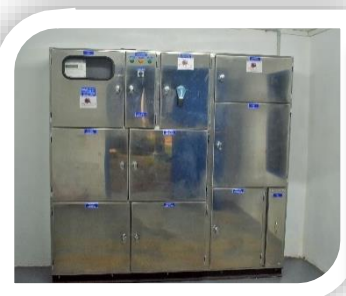
Figure 5. Savusavu WTP main switchboard
