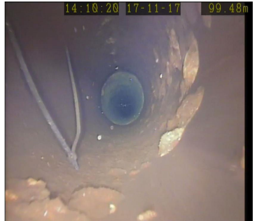
Biological Build up (and cable tie)
